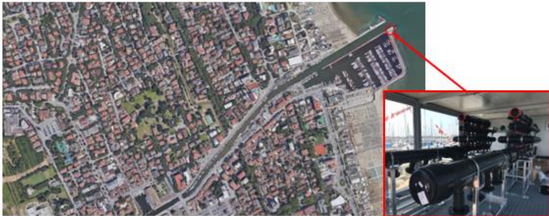
Figure 5: The installation in the harbor of the municipality of Cervia. In particular, a detail of the two autopurging disk filters within the cabin is shown.
